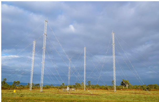
Babcock's Defence High Frequency Communications System (DHFCS), an Australian sovereign capability providing long-range secure and non-secure tactical voice communications.
